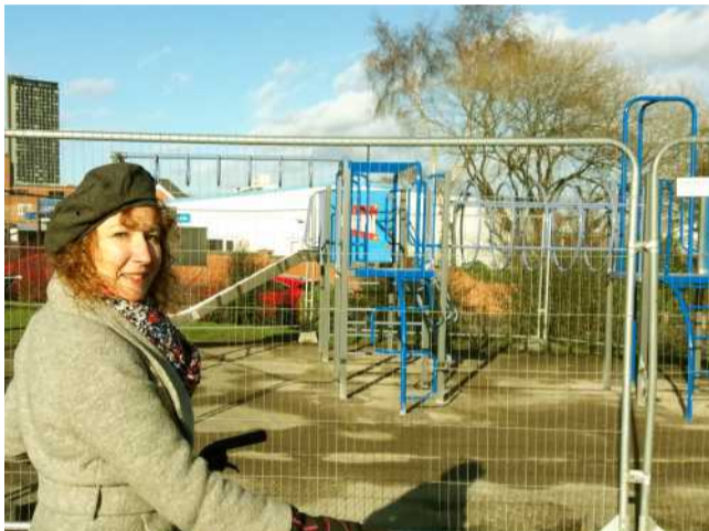
Cllr Ruth Mersereau checking progress of work at Duchess Road Pocket Park
