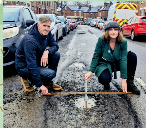
Calling out poor pothole repairs and pushing for action
