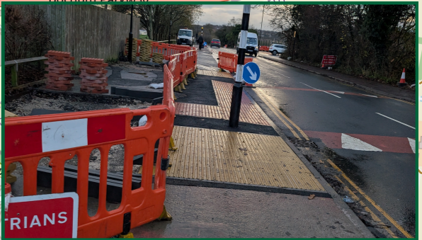
Secured the prompt resurfacing of the new crossing by Meadowhead School after a resident was injured
