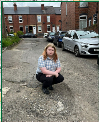
Started a petition to get Osmaston Road adopted and resurfaced
